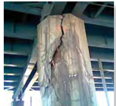
Philadelphia pier crack. Photo courtesy of Pennsylvania Department of Transportation.
