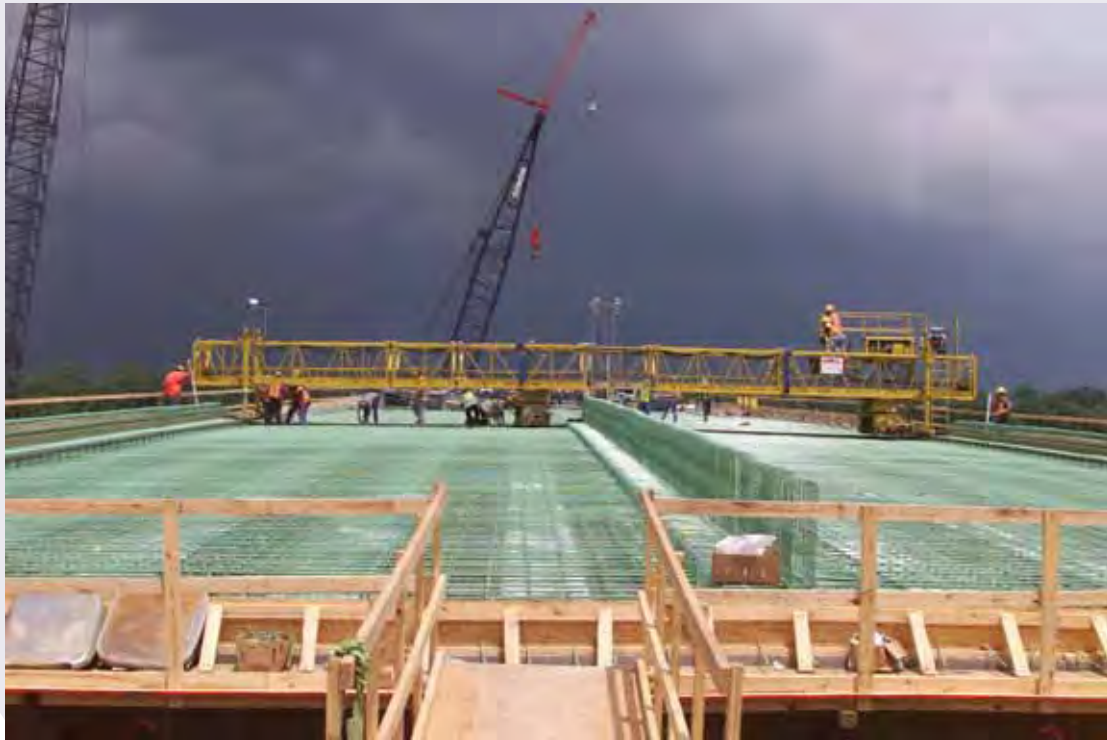
Reconstruction of the Interstate 40 Bridge in Webber Falls, Oklahoma after it was damaged by a runaway barge. Photo courtesy of Oklahoma Department of Transportation.
