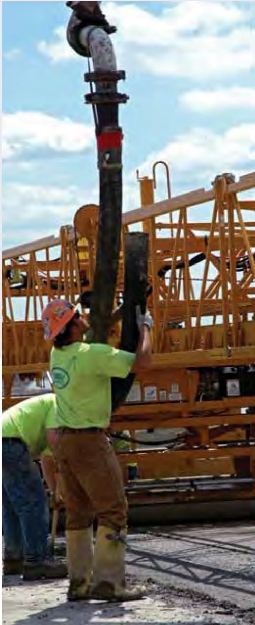
Workers operate concrete pump in the building of the I-94 Business loop of Memorial Bridge North Dakota. Photo courtesy of Mike Kopp, North Dakota Department of Transportation, 2008.
