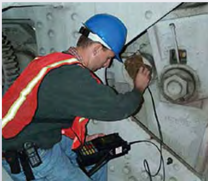
An engineer tests a bridge pin using ultrasonic technology. Photo courtesy of Federal Highway Administration.
