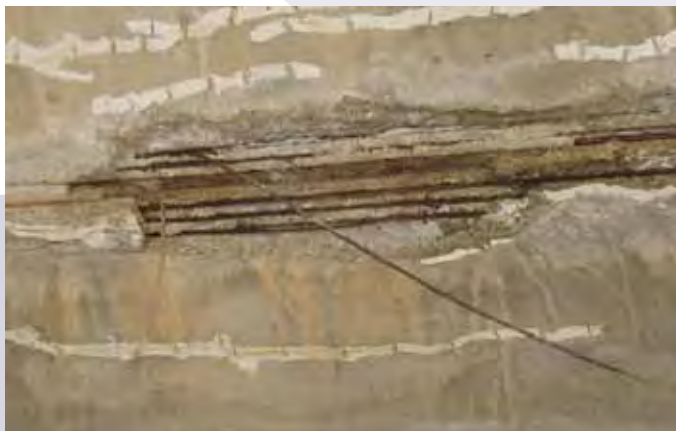
I-25 deteriorating girder.
