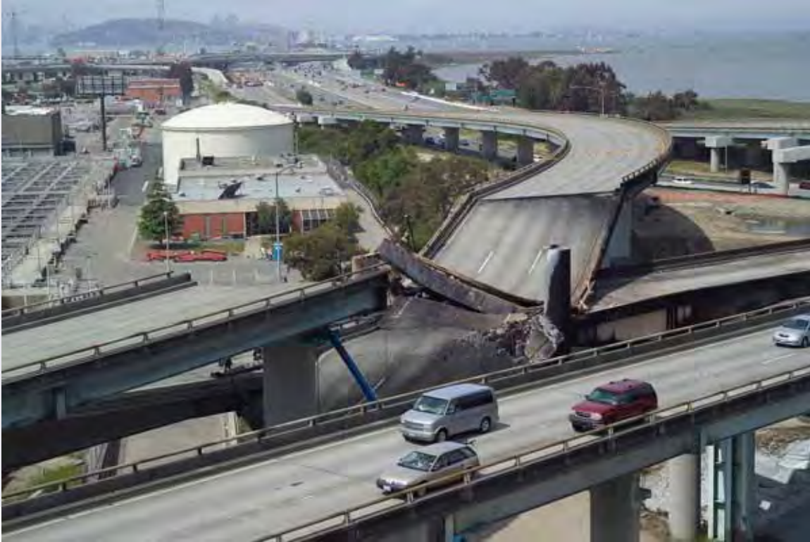
Damage to MacArthur Maze overpass. Photo courtesy of Caltrans.
