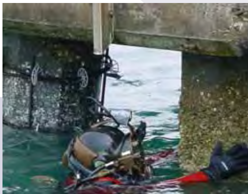
A diver inspects a bridge piling. To the left, the diver has placed steel rebar, which reinforces the bridge’s concrete piling, around the pressure-washed and cleaned piling. A new pile jacket will be placed around it.
