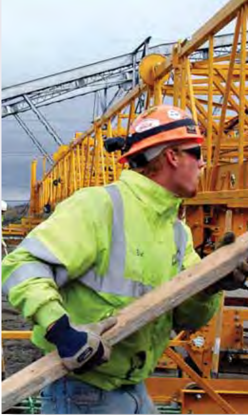
Worker on site of I-94 business loop construction of Memorial Bridge North Dakota. Photo Courtesy of Mike Kopp, North Dakota Department of Transportation.
