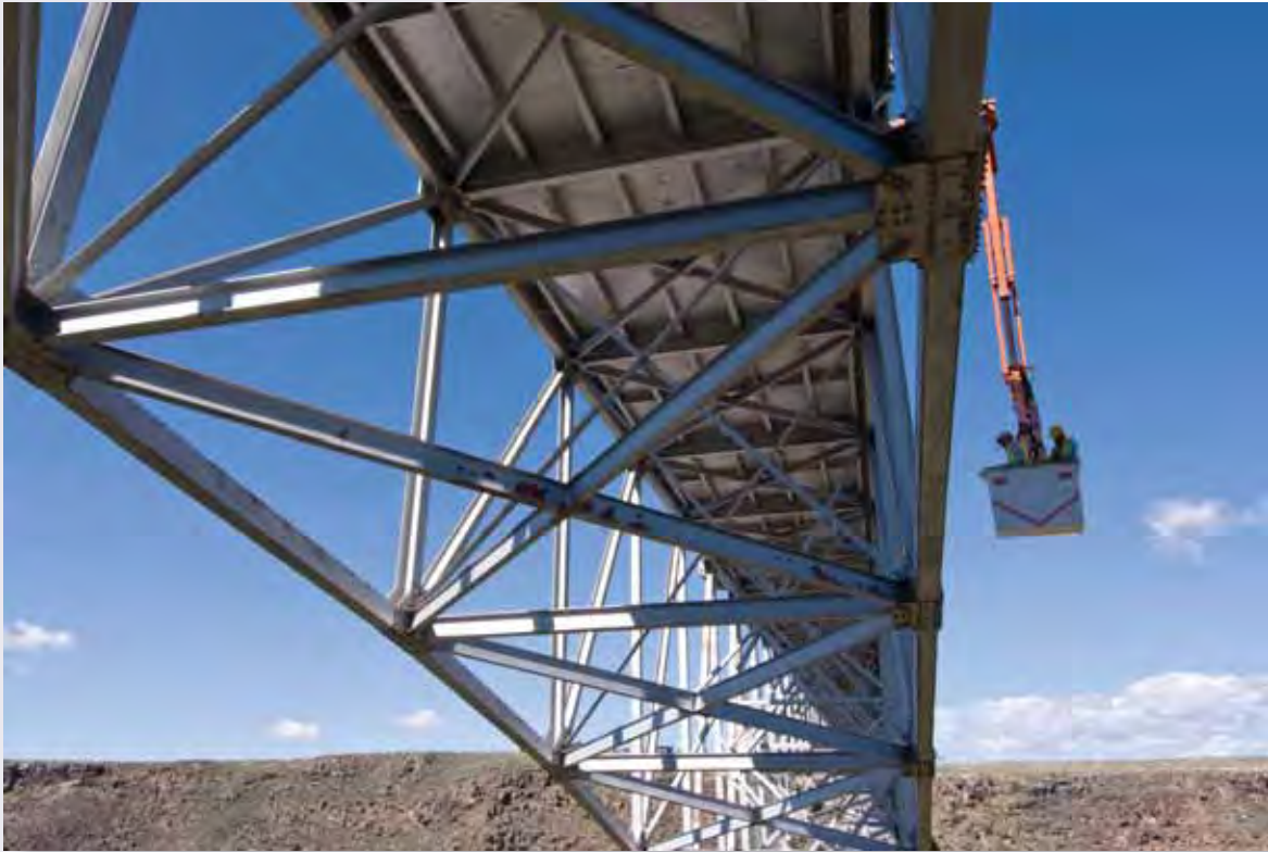
The Rio Grande Gorge Bridge being inspected after the I-35W bridge collapse in Minneapolis. Photo courtesy of New Mexico Department of Transportation
