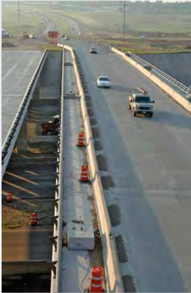
Construction and completed bridges at intersection of Interstate 35 and Loop 340 in Waco. Photo courtesy of Stan A. Williams, Texas Department of Transportation.
