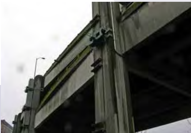
Seismic retrofit bridge: a viaduct in Washington State. Photo courtesy of Washington Department of Transportation.
