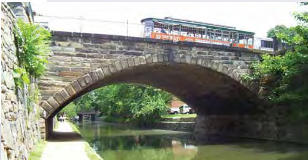
The Chesapeake & Ohio Canal flows under the stone masonry arch of the Wisconsin Avenue Bridge in the busy Georgetown area of Washington, DC. The towpath beside the canal serves as a footpath and recreation resource. The original wrought-iron railing dates back to 1831.
