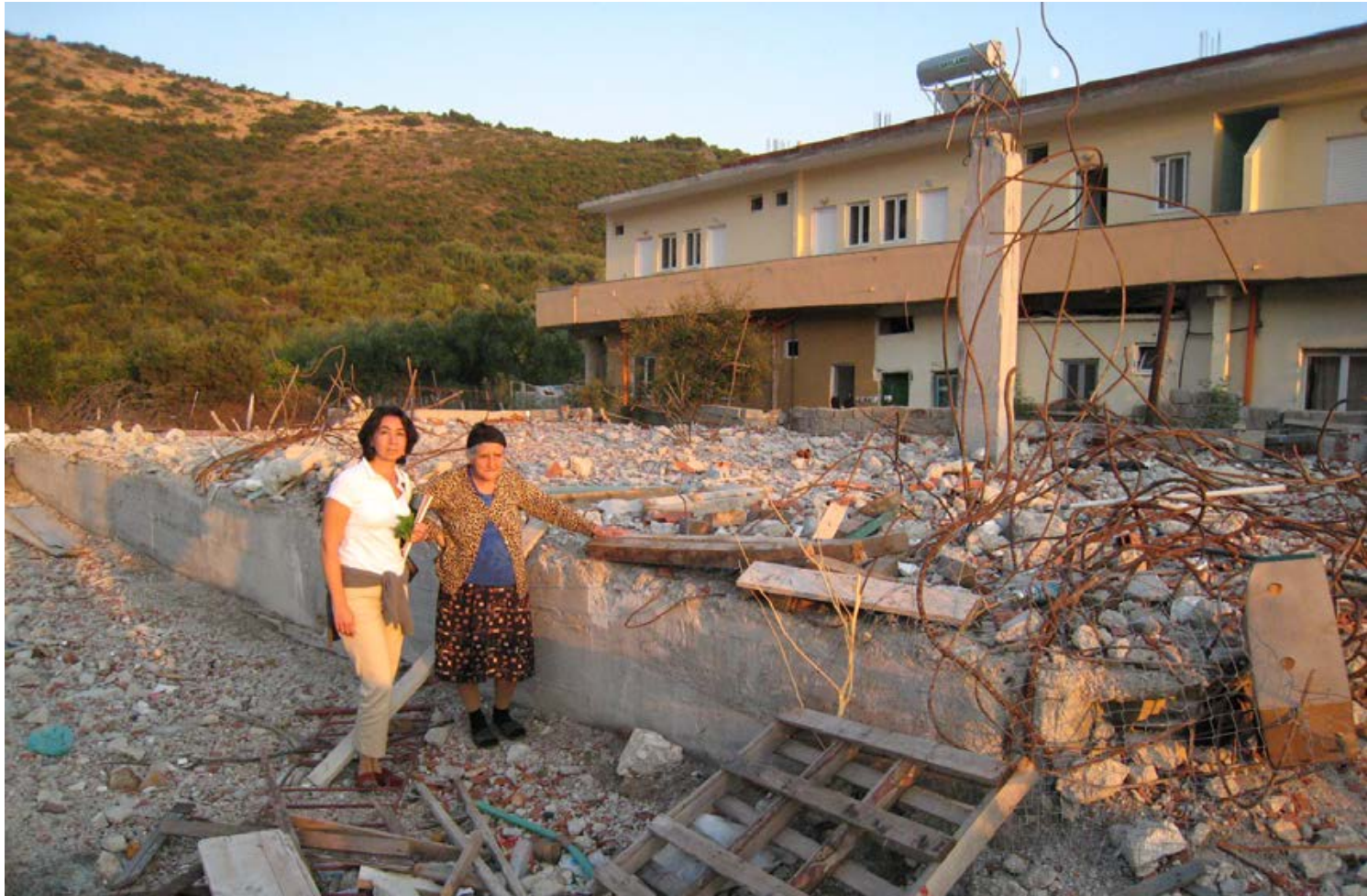
Dilek Barlas, left, then the Panel's deputy executive secretary, with a Requester in front of her demolished property as part of the investigation of the Integrated Coastal Zone Management and Clean-up Project in Albania.
