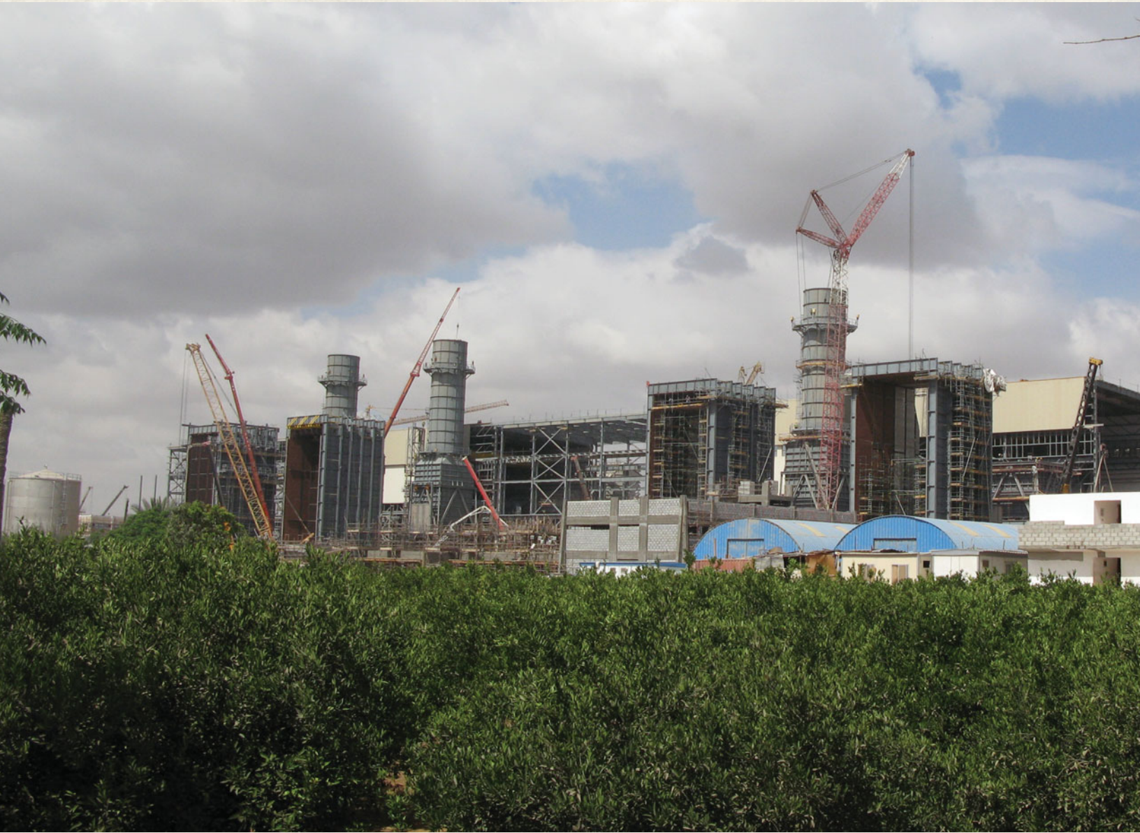
Giza North Power Plant seen from one of the farms, Giza North Power Project, Egypt.
