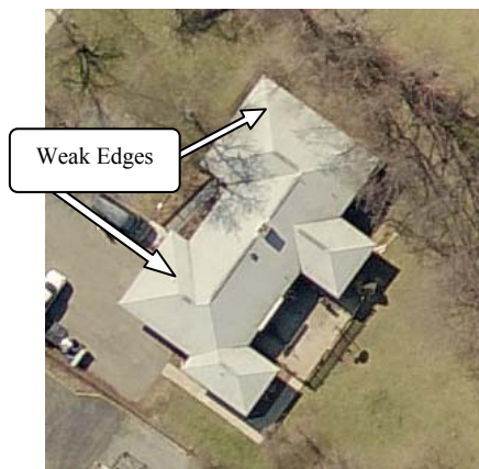
Figure 1. Weak edges of roof's ridges
