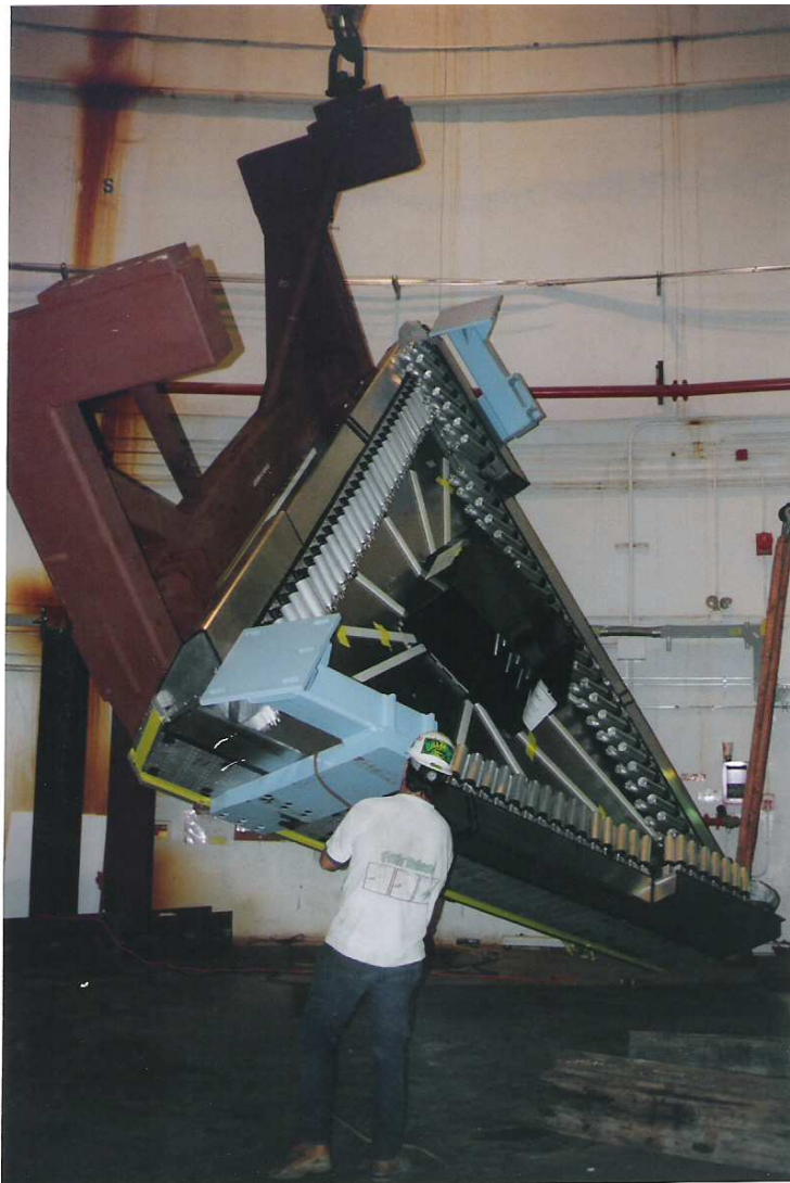
Figure 10.7: Photograph of the EC tooling used to lift and install the CLAS EC sectors.
