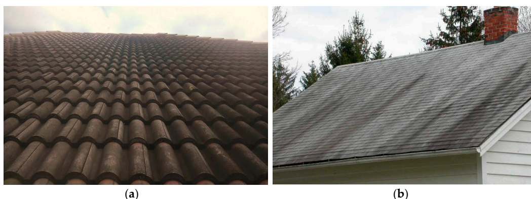
Figure 1. (a) Mould growth on concrete tiles; (b) Mould growth on asphalt roofing shingles.
