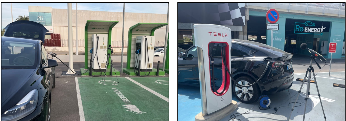
Figure 4. Ingeteam 50 kW fast charging station (left) and Tesla V2 Supercharger 150 kW (right).
