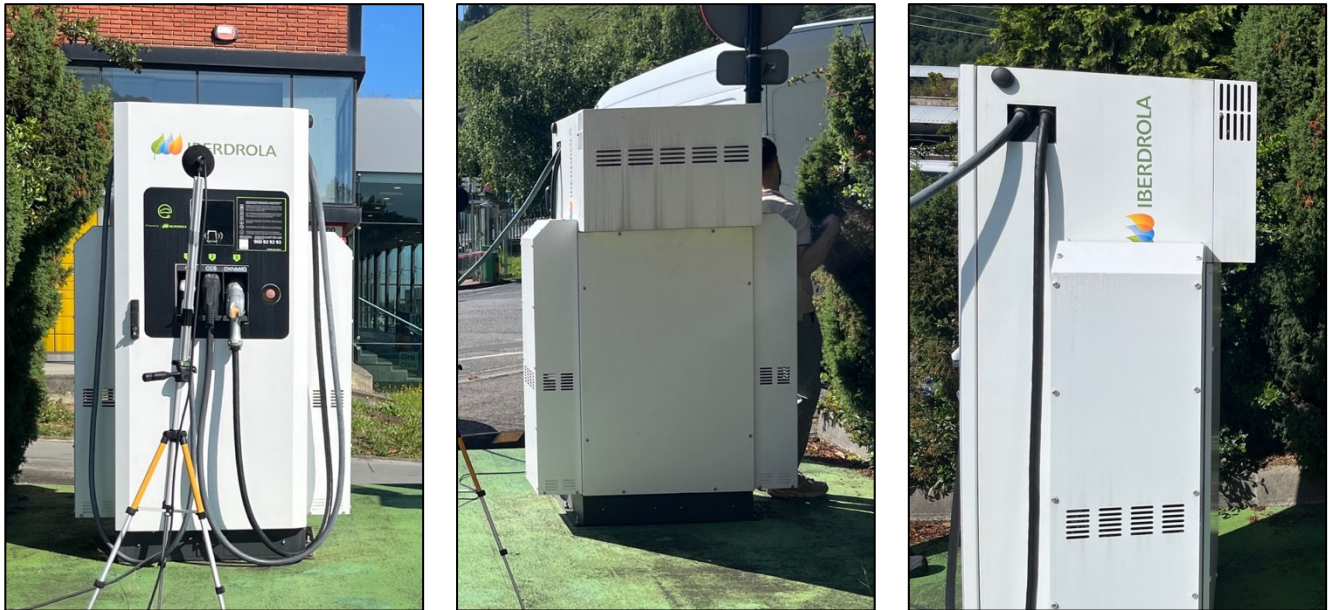
Figure 10. Ingeteam Rapid 50 kW fast charging station with a sound-dampening device.
