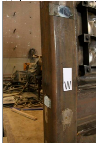
(c) External buckling of column walls
