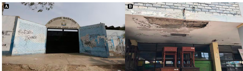
Figure 4. (A) State educational center in Lima lacking adequate infrastructure reprinted with permission from Ref. [28]. 2018, Hugo Pérez and El Comercio; (B) School with roof damage, reprinted with permission from Ref. [28]. 2018, San Juan de Miraflores Municipality.
