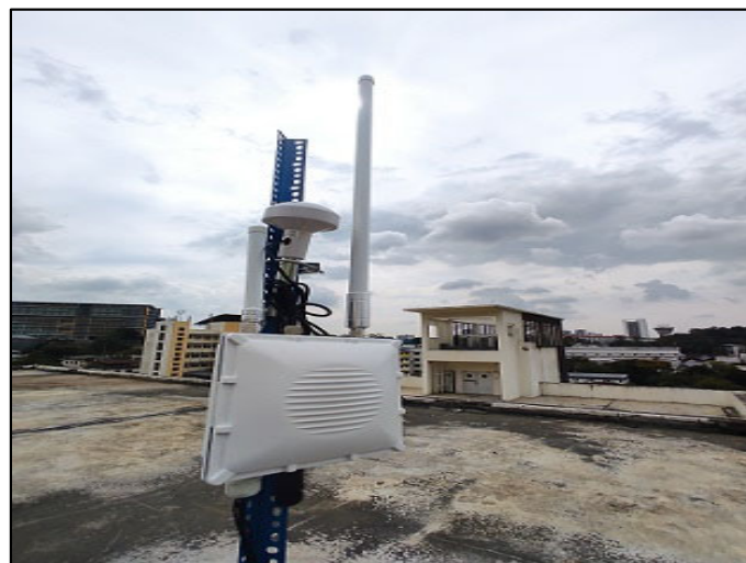
Figure 5. LoRa gateway positioned on the rooftop.
