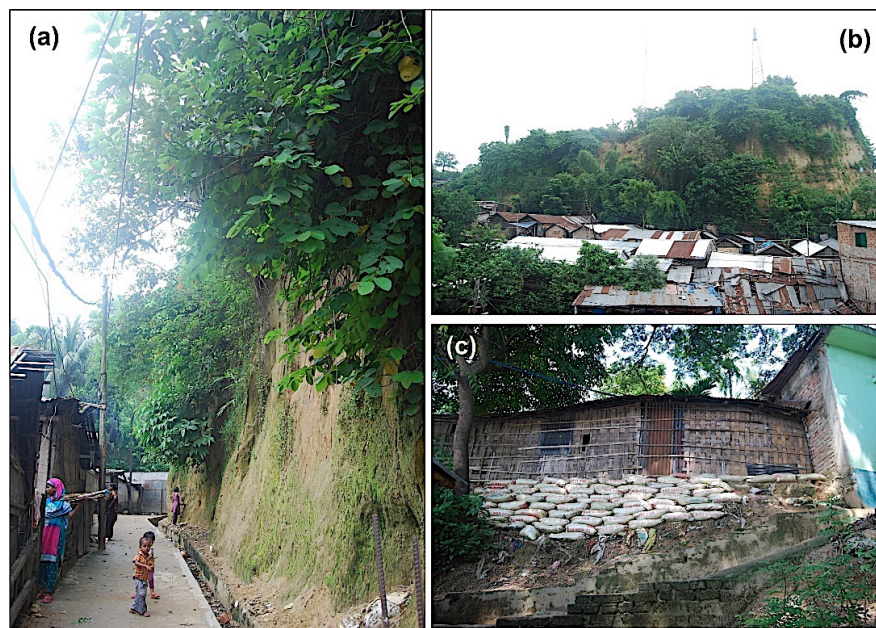
Figure 12. A cluster of houses built on dangerous foothills by cutting hills, where people are living under serious threats of landslides in CMA. Source: Bayes Ahmed, fieldwork, 2015.
