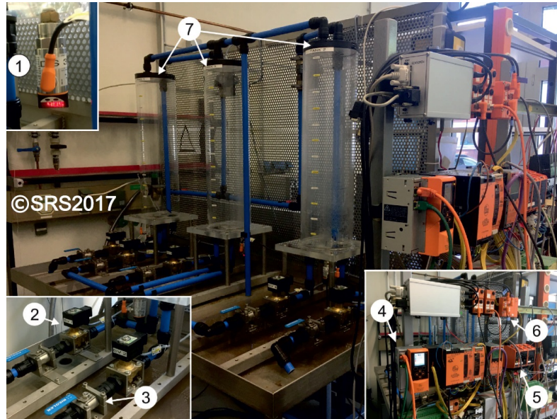
Figure 2. Test rig of the 3TS at the Chair of Dynamics and Control (SRS) at the University of Duisburg-Essen (UDE): (1) pressure sensor, (2) two-way switch valve, (3) ball valve, (4) programmable logic controller, (5) digital/analog module, (6) analog/digital module, and (7) tanks [28].
