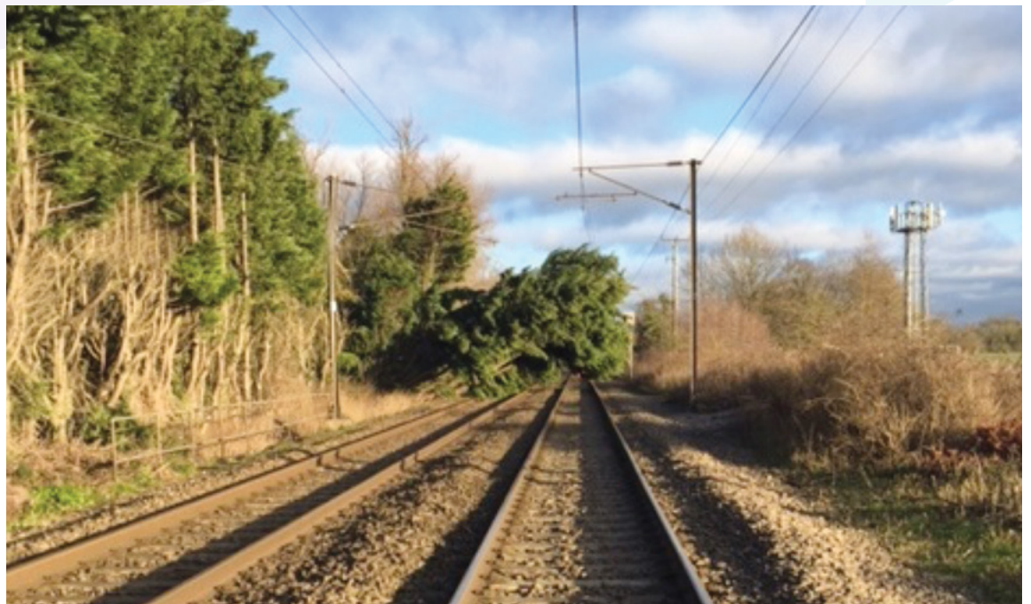
Figure 9 Fallen tree (wind damage) causing a dewirement near miss, January 2018
