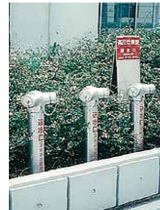
連結送水管 Connecting Water Supplying Pipe
