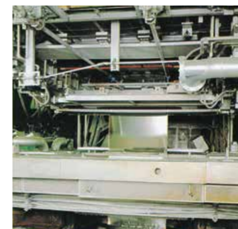
溶融亜鉛めっき設備 Continuous Galvanizing Line
