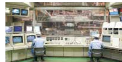
No.2溶融亜鉛めっき設備の運転室 Operations room of No.2 Continuous Galvanizing Line
