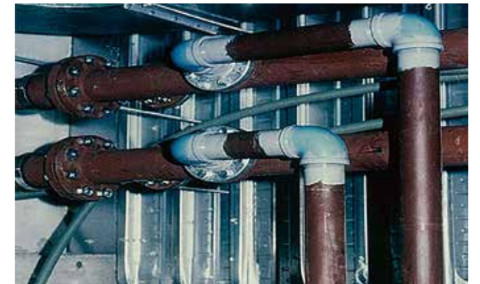
屋内給水配管 Water Supply Pipe Line
