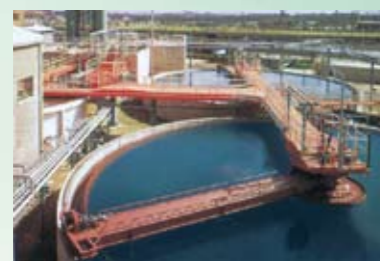
廃酸処理設備 Waste acid treatment facility
