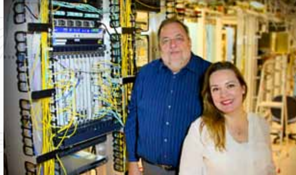
SDSC Network Architect Thomas Hutton and Christine Kirkpatrick, SDSC's division director of IT Systems and Services, stand beside one of the campus' Juniper MX960 routers. The system, which has speeds as fast as 100 Gb/s, provides the main Internet connection to UC San Diego, SDSC, and the UCSD Medical Center.
