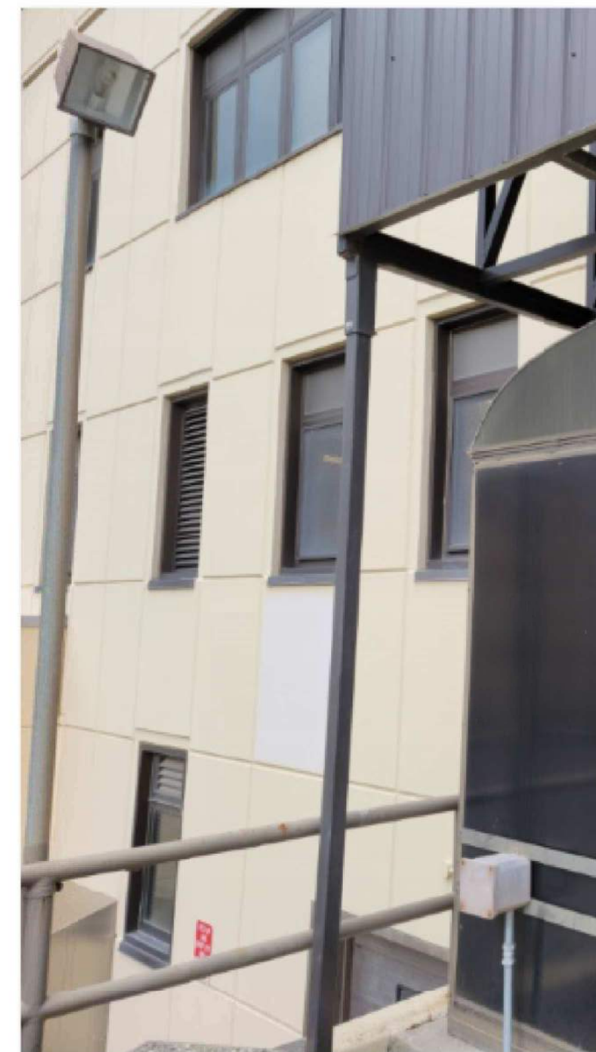
EXISTING LIGHT POLE AND POTENTIAL PANELBOARD SPLICE POINT
