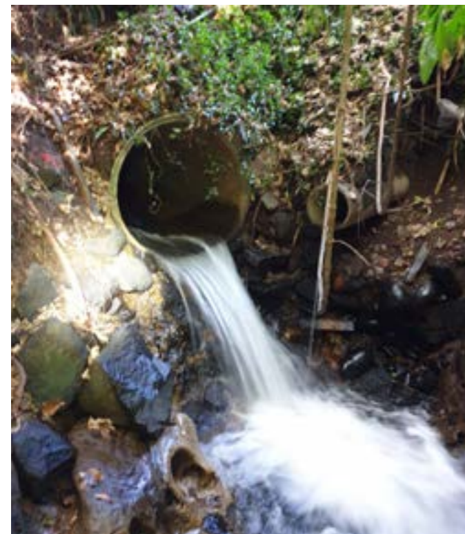
Non-compliant stream culverts can prevent the upstream migration of fish due to the swift flows, shallow flows, steep approaches (waterfalls), overhangs (or perches) and by not providing rest areas.
