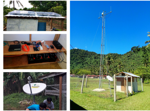
Figure 5: Components of a typical UP CCN installation: solar panels (top left), battery bank and network hardware (middle left), VSAT antenna (bottom left), outdoor GSM radio system, tower and shelter (right).
