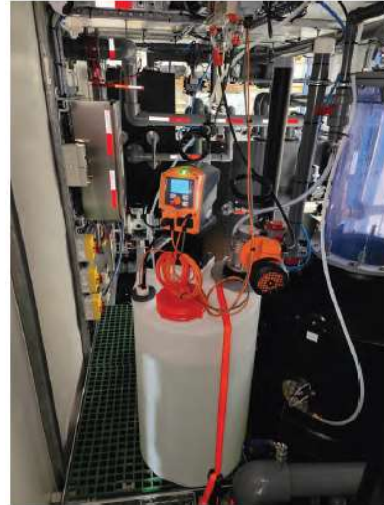
Figure 20: Dosing tank and pump
