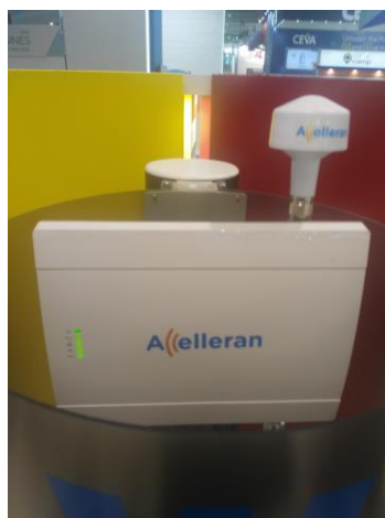
Figure 24 - Accelleran E1000 Series inside 5GCity Showroom Lamppost
